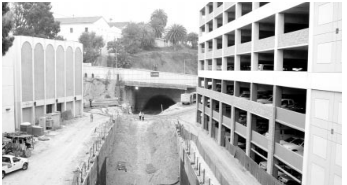
On October 5 workers punched through the wall separating the two trolley tunnel segments under campus.
